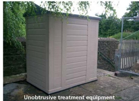
Unobtrusive treatment equipment
